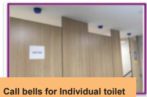
Call bells for Individual toilet cubicles improved safety for the elderly in the event of falls
